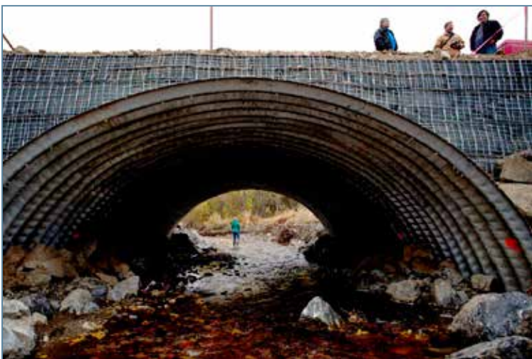
A fish-friendly culvert in Tyonek, Alaska. Photo by Ash Adams.
