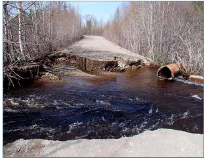
A small round culvert that failed during a 2012 flood event. Photo from USFW.
